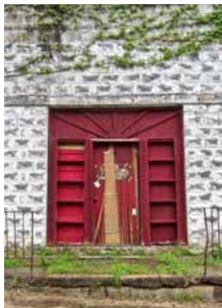
A damaged door sign discourages trespassing in Calico Rock.
