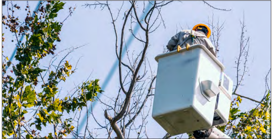
First Electric's right-of-way crews work year-round on vegetation management. The co-op also uses outside contractors to help with maintenance. Clean-up crews usually follow three to five days after maintenance.
