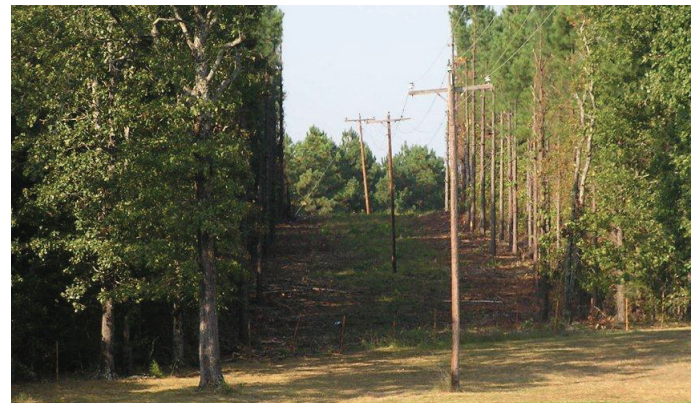
First Electric maintains our rights-of-way in an effort to keep members of the public safe and to help minimize outages.
